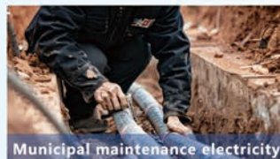
Municipal maintenance electricity
