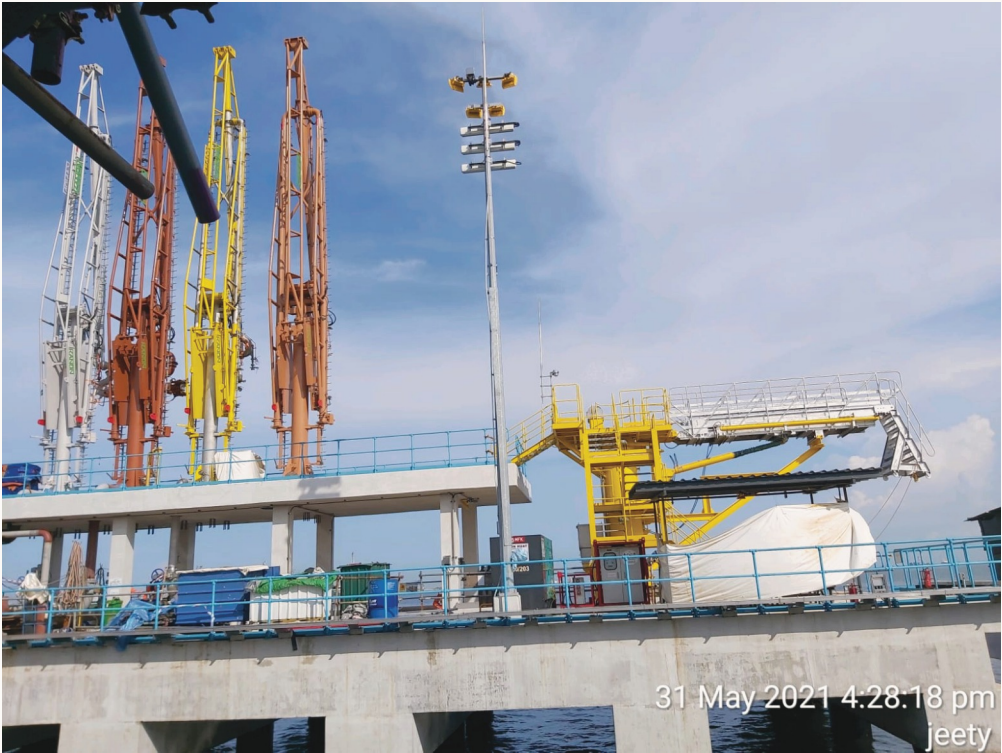
Lighting / Power /Lightning Installation
