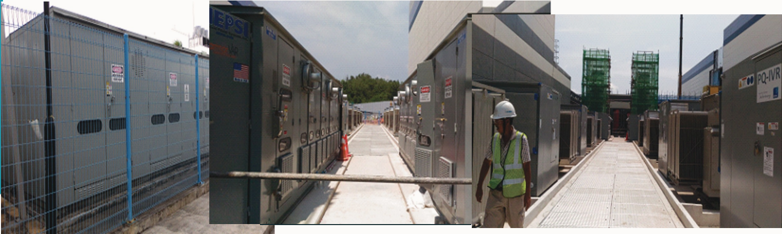
High Tension Switchgear and Transformer Micron Fab 10 Extention (Fab 10X) F11D
