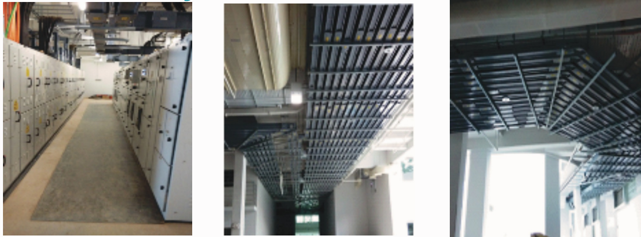
Low / Middle Voltage Switchboard and Busduct
