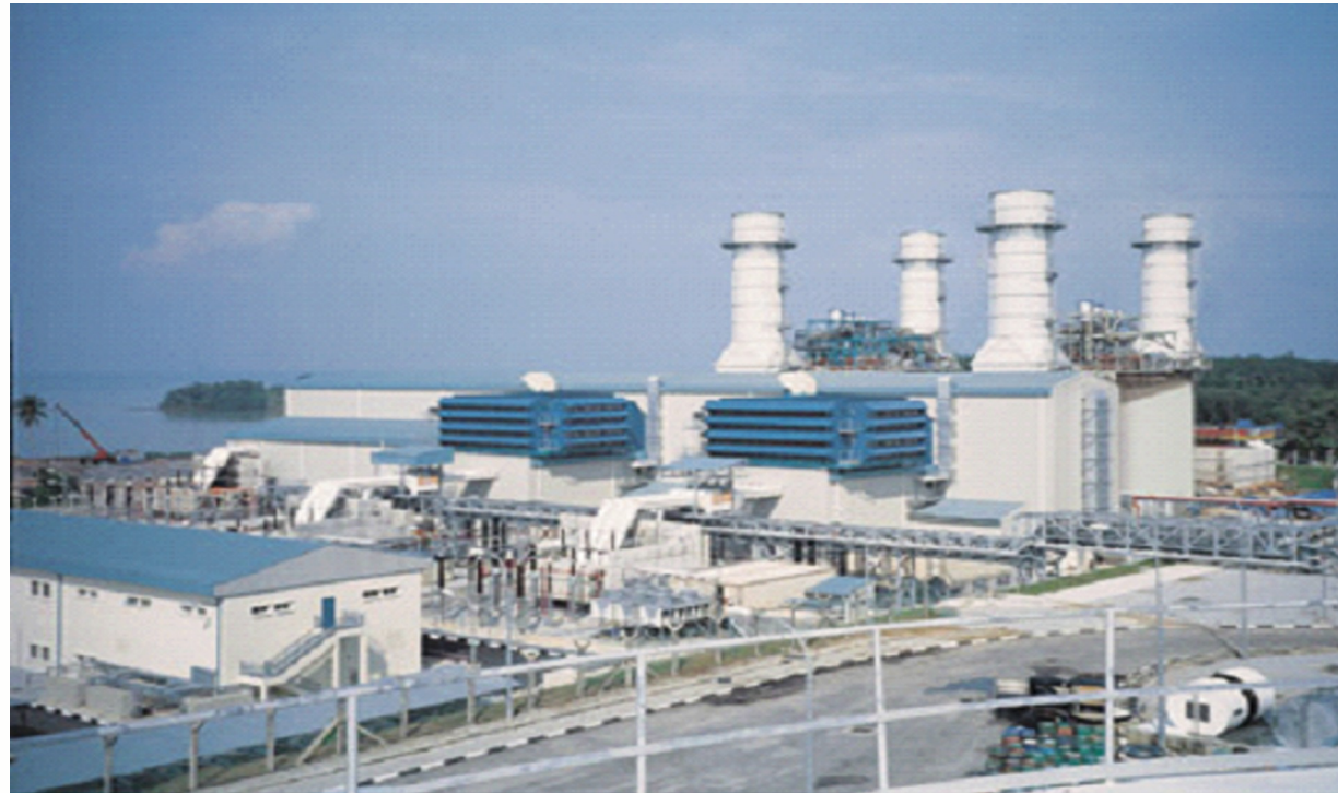
720MW COMBINED CYCLE POWER PLANT – PANGLIMA @ MELACCA
